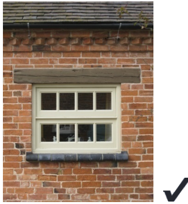
Fig 3: Retained timber lintel and chamfered blue brick cill. This size of window opening should normally be filled with an inward opening hopper-style window
