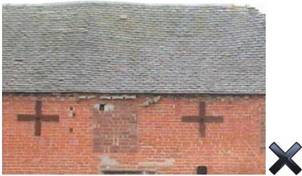
Fig 4: Window infilled incorrectly
