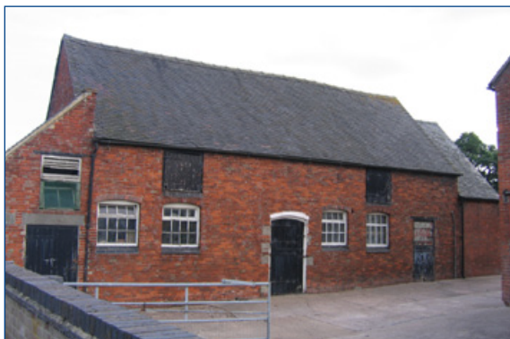
Many cowhouses were converted from earlier barns and other buildings in the late 19th and early 20th centuries. The windows to this range have been inserted, and the metal frames conform to 1930s hygiene regulations.
