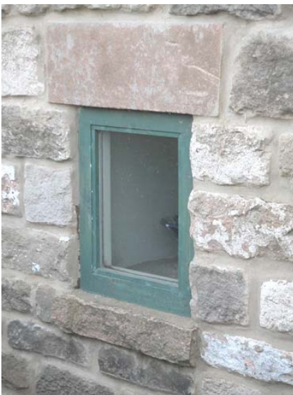
7: Flush rubbed pointing and simple window style : the muted colour is sympathetic to the vernacular style of building
