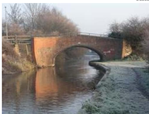
Trent and Mersey Canal Bridge 29 (Photographs reproduced by kind permission of Liz Winson)
