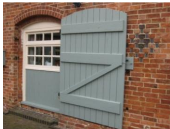
Fig 2: Retained redundant door with the window recessed in the opening. Top-hung opening lights as shown in this picture will generally not be acceptable as they are not a traditional detail.
