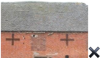
Fig 4: Window infilled incorrectly
