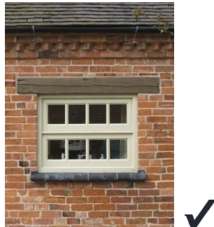
Fig 3: Retained timber lintel and chamfered blue brick cill. This size of window opening should normally be filled with an inward opening hopper-style window
