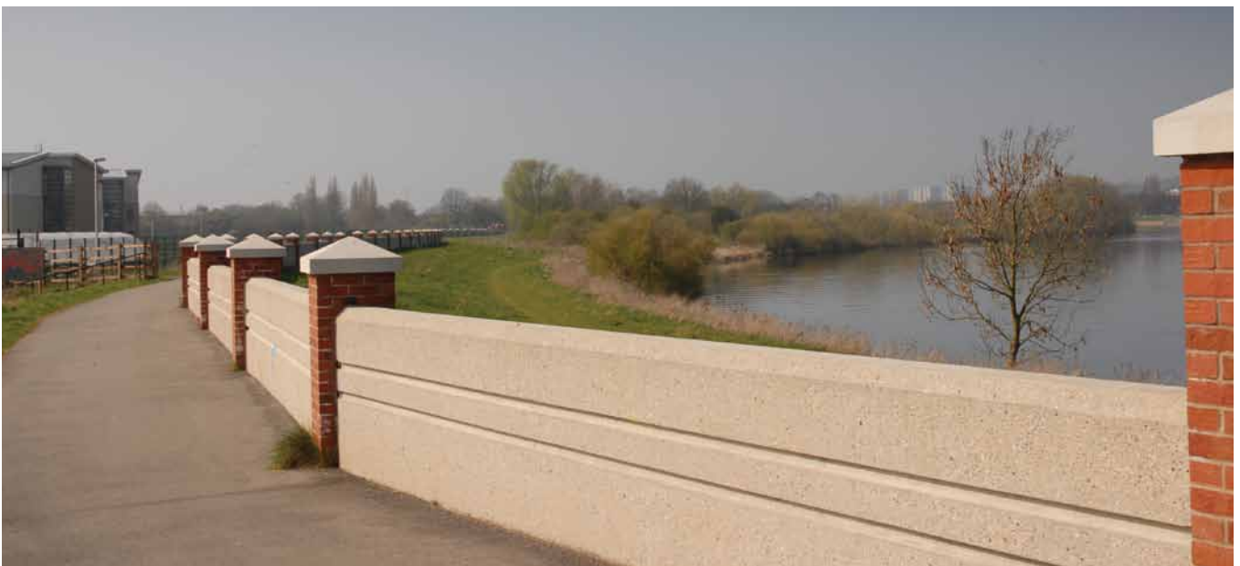
↑ Flood defence scheme, West Bridgford
